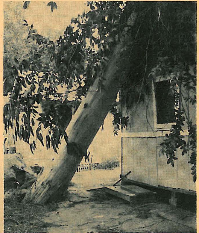
WEEKEND HIGH WINDS MOVED THIS TREE ONTO ONE OF THE SMITH COTTAGES LOCATED OFF OF HWY. 80. THE NEW RESIDENT WAS SURPRISED, BUT FORTUNATELY WAS NOT INJURED. (Town and Country Photo)
